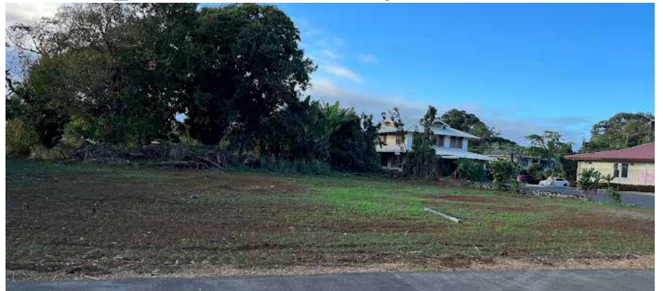
Wally Andrade recently donated crew and dozer to clear land along Hwy 11 next to Hawai'i Island Community Health Center's Ka'ū Family Health & Dental in Nā'ālehu. OKK hopes to put in a dialysis center. Photo from OKK
