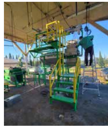
The new wet mill at Ka'ū Coffee Mill will process 10,000 lbs. an hour. Photo from Ka'ū Coffee Mill
